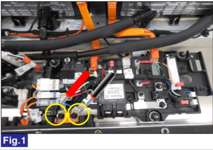
Fig.1) Measuring capacity between inverter (+) and inverter (-)
